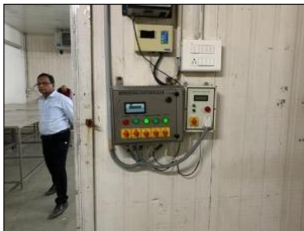
Ripening chamber controller, Export facility centre, Talegaon Dabhade
