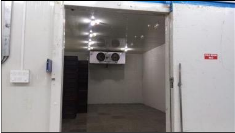
Cold storage Export facility centre, Atpadi
