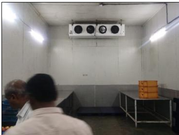
Cold storage, Vashi
