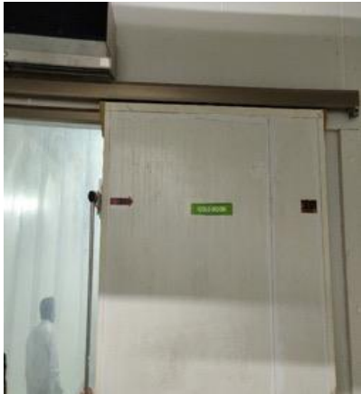
Cold storage, Export facility centre, Karmad
